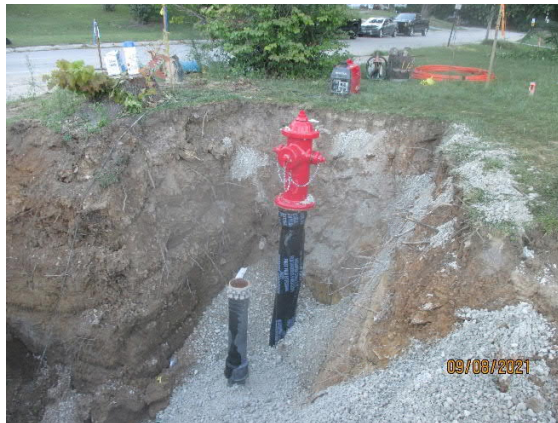
View of installed fire hydrant and 6" valve near Sta: 221+88 RT.
